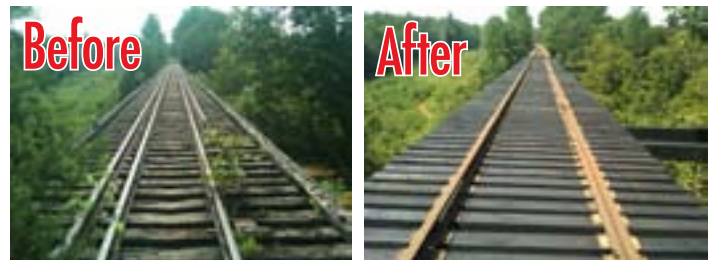
Before and after: The South Fork River bridge was upgraded with new ties and 132-pound jointed rail.
