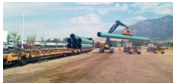
Providing on-time, reliable rail service is crucial for the project's success, as contractors must be called in to off-load pipe when the train arrives.
